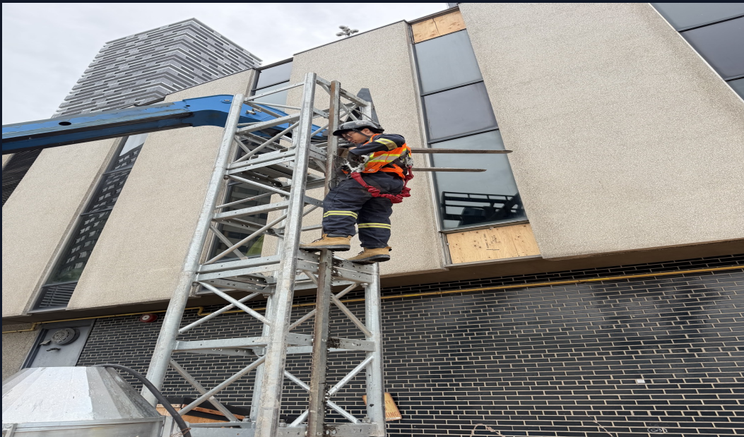
Licensed EDMB mechanic on platform
